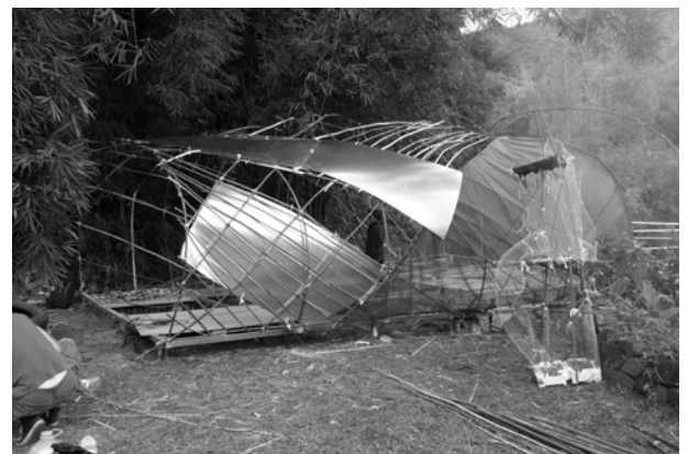
Figure 4 - Gastronomica The Gastronomica room nearly finished is partially sheltered by giant bamboos on one side and is framing the large landscape on one end. Courtesy: René Paul Savignan.
