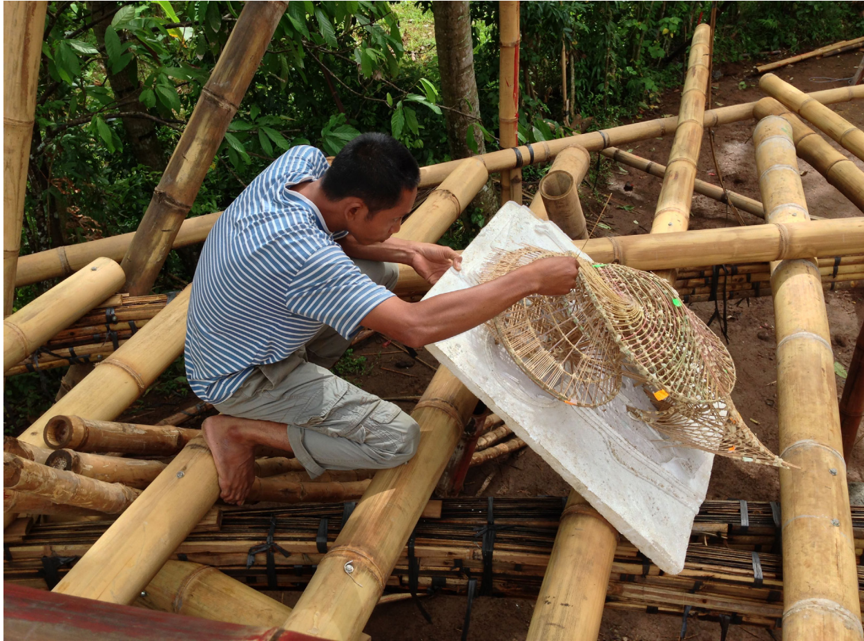
Figure 7: The construction is executed by scaling directly from the 1:50 model in the field (©Ibuku) courtesy of Elora Hardy / Ibuku.
